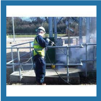
Effluent Treatment Plant Service
