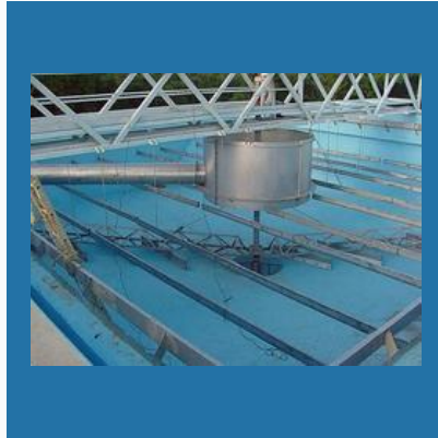
Water Treatment Clarifier
