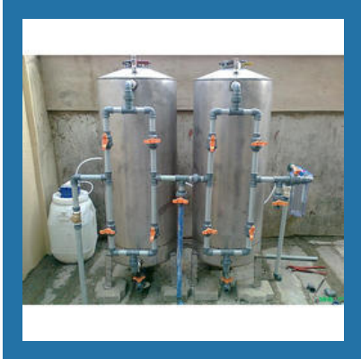
Grey Water Treatment Plant
