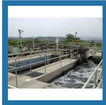
Industrial Sewage Treatment Plants
