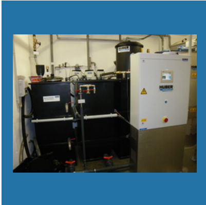
Greywater Treatment Plant
