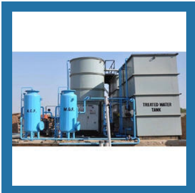
Waste Water Purification Plants
