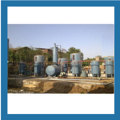
DM Water Plant
