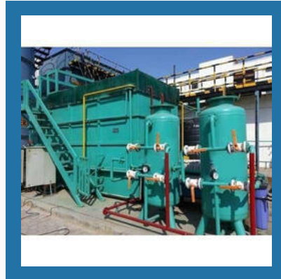
Industrial Effluent Water Treatment Plants
