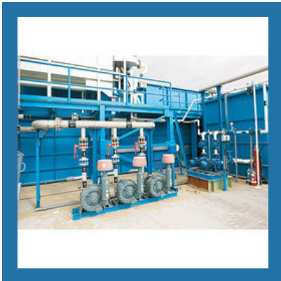
SAFF Technology Based Sewage Treatment Plant
