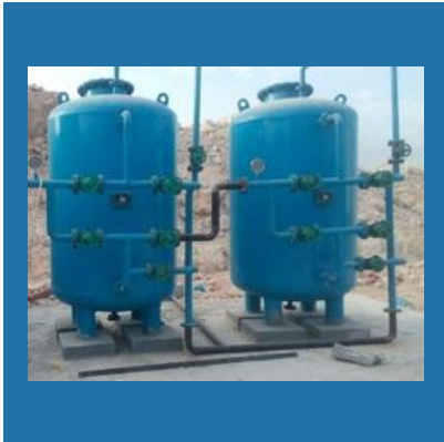
Groundwater Treatment System
