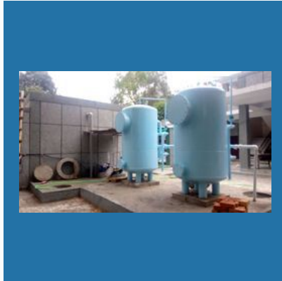
Conventional Sewage Treatment Plant
