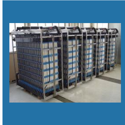
Membrane Bio Reactor
