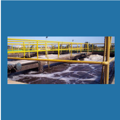
Extended Aeration Technology Based Sewage Treatment Plant
