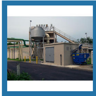
Grey Waste Water Treatment Plant
