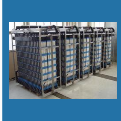
MBR Waste Water Treatment Plant
