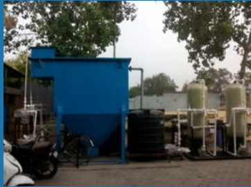
Packaged Effluent Treatment Plant
