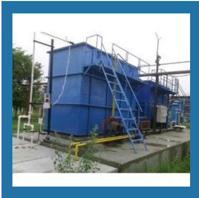
STP Plant For Hospital
