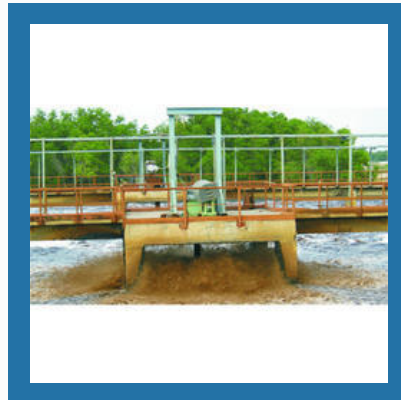
ETP Filter Presses
