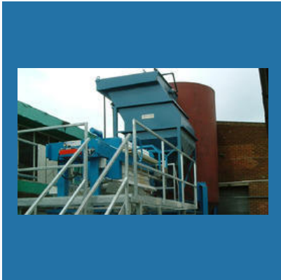
Effluent Treatment Plant for Distillery
