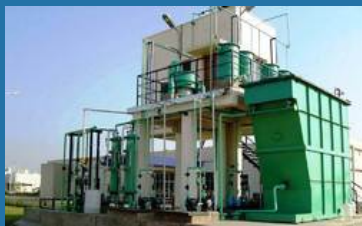
Sewage Treatment Plant For Hospital
