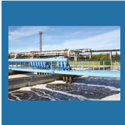
Industrial Wastewater Treatment System
