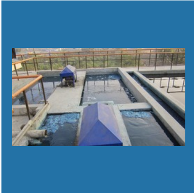
Effluent Treatment Plant for Textile industry
